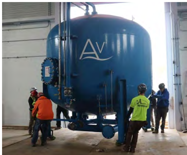
PFAS Treatment Vessel
